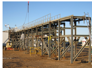
Top level pipe racks for Jones Act Tankers.
